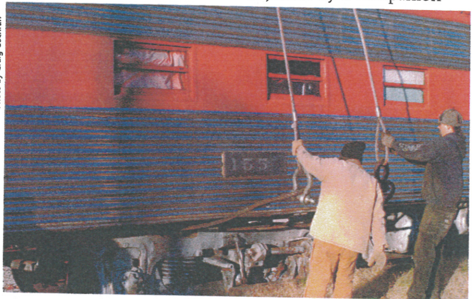
Heavy steel cables were used to hoist the car, which was thoroughly checked out by IAM railroad experts prior to its journey to Chicago.
