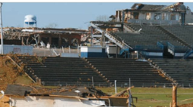
Hardest hit was Enterprise High School, where eight students died when the tornado collapsed the building's cinder block walls.
